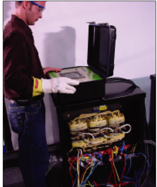
MEASURING THE INSTALLED EFFICIENCY & POWER QUALITY OF A TRANSFORMER.
